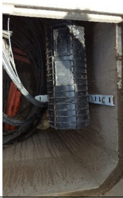
Figure 15. Splice case at Pennington Vault
