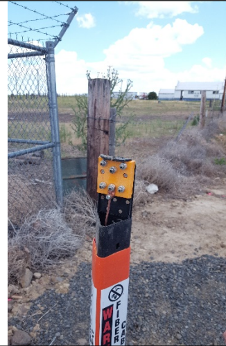
Figure 12. Marker for CBEC Spliced Vault
