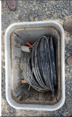
Figure 13. 50 ft. of Slack for Spliced Vault
